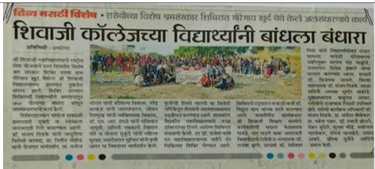
Students of our college constructed small bunds to store water and increase water level.
